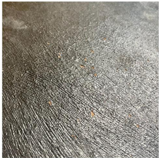
Figure 4: Area of cupping paint after treatment.
