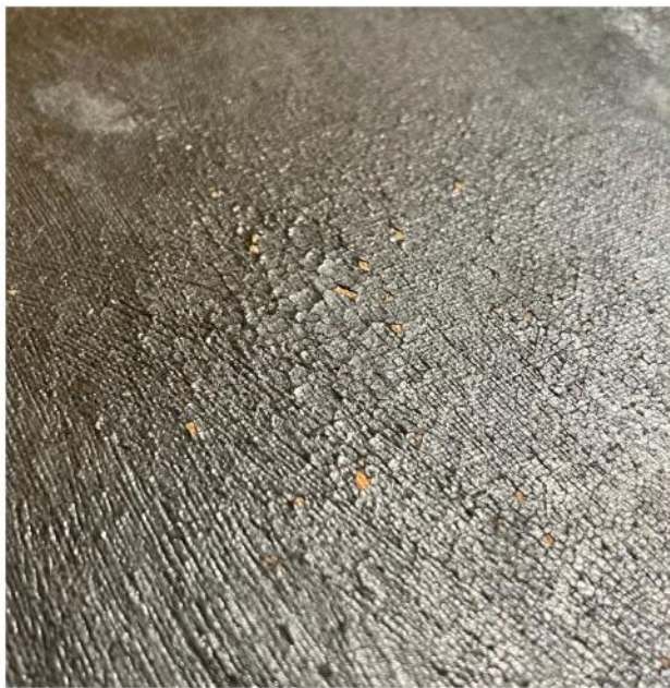
Figure 3: Area of cupping paint before treatment.
